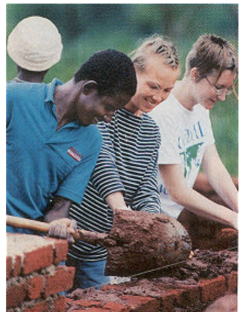
In Tanzania in '99, a Global Volunteers group constructed a latrine for a dorm.
